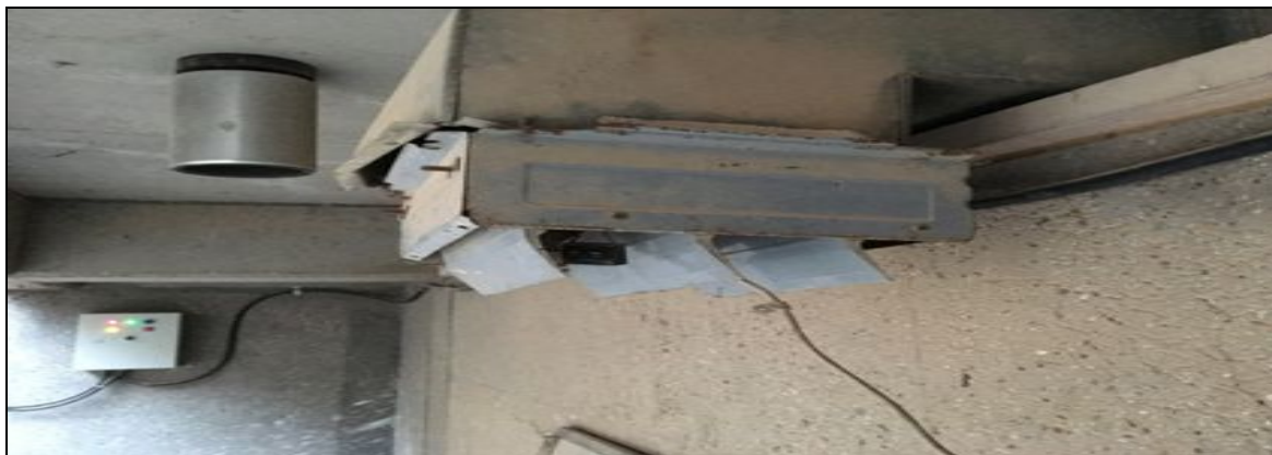
Figure 1. Side view of a small fan fixed directly to the upper windows that made up the old ventilation system
