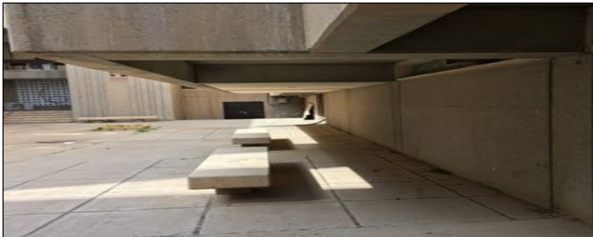
Figure 3 In the old system, the exhaust was routed directly into the student movement area
