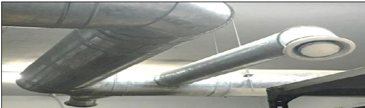
Figure 5. Close-up of ventilation ducts.
