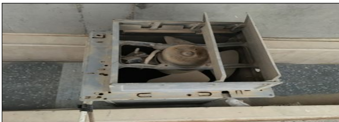
Figure 2. One of the small fans fixed directly to the upper windows that made up the old ventilation system
