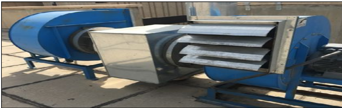
Figure 8: Close-up of alternating fans.
