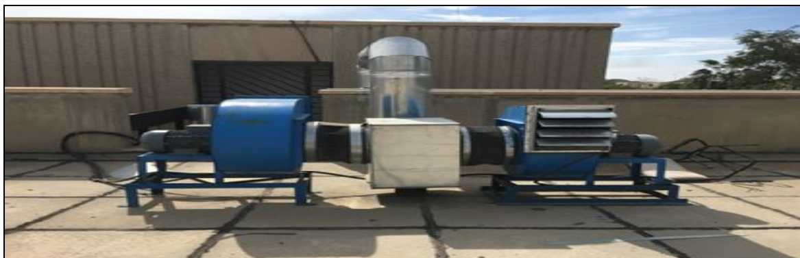
Figure 7: Two alternating fans have been installed.
