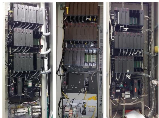
Fig. 1b. MOSCAD-RTU cabinets
