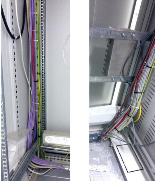
Fig. 6. Cable harnesses entering the communication cabinets through the floor opening
