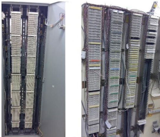
Fig. 1c. Digital Distribution Frame (DDF) and Main Distribution Frame (MDF). Left – installed in the cabinet, right – wall-mounted open panel.
